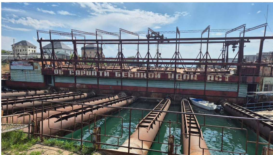
Somgor-1 floating pumping station
